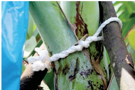
A Prop is Two Poles Tied Loosely Together
