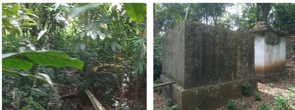
Figure 8: Main Pipeline and the pump house at Dodangolla
