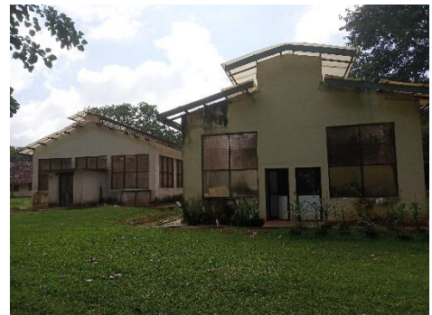
Figure 5: Glass houses in dilapidated condition
